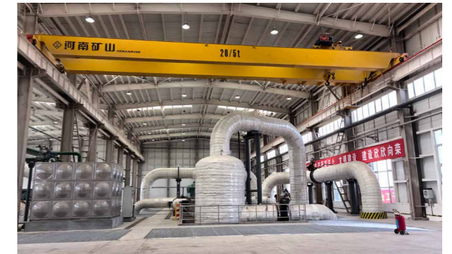
The Tuoketuo Power Plant-Hohhot long-distance heating pipeline
