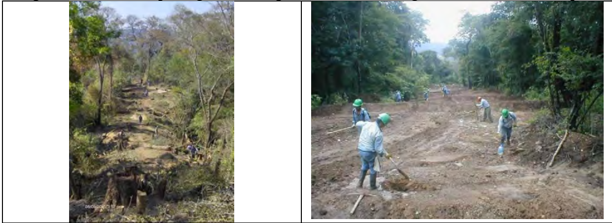
Figures 1a and 1b. Opening and closing narrow ROW using labor intensive technique 7
