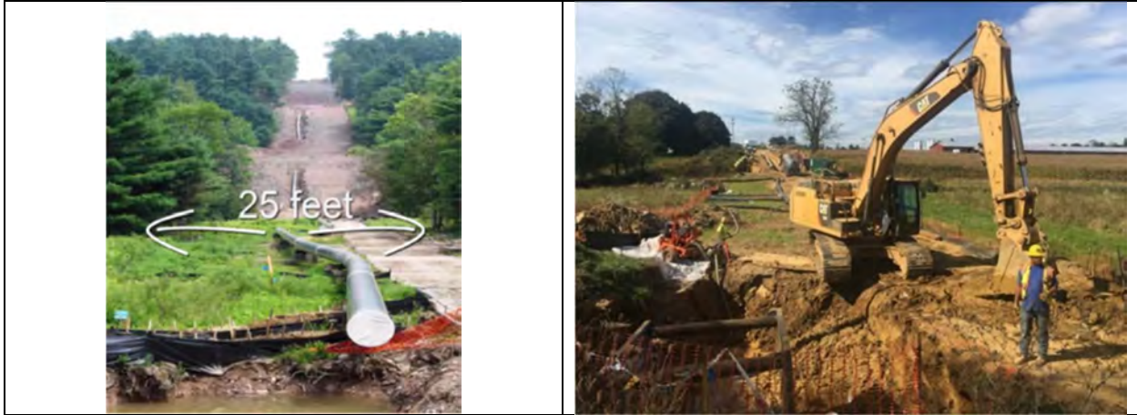
Figures 2a and 2b. typical Pennsylvania 15-meter pipeline ROW (25 feet on either side of centerline), 8 and clearing of ROW for 20-inch diameter Mariner East Pipeline 9
