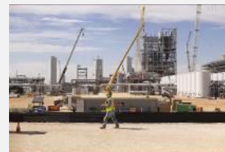
STRATOS, the world's largest direct air capture (DAC) facility Photo courtesy of 1PointFive, a U.S. company
