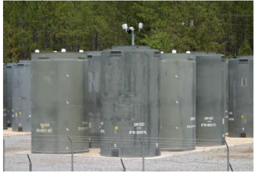
Dry storage at Plant Hatch.
