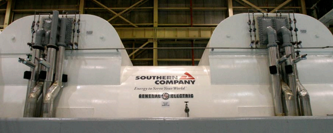
Plant Hatch's Unit 1 Generator
