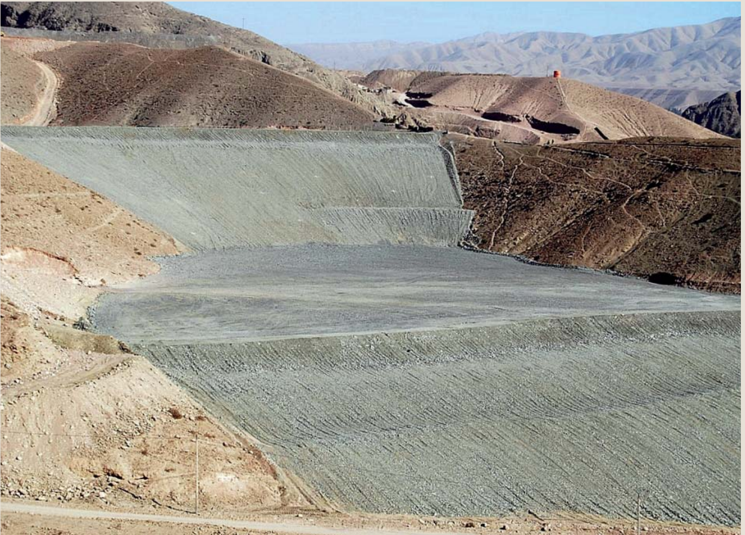
Candelaria and Ojos del Salado voluntarily covered and stabilized three of their old tailings storage facilities.
