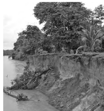
River bank erosion caused by flood
